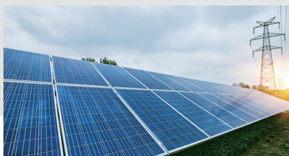
Solar energy panels
