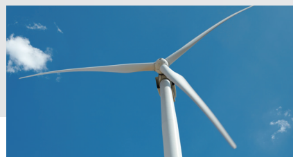
Wind powered turbines
